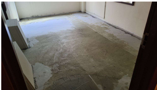
Photo 3.29: Photo of the base coat that have been applied to the floor.
