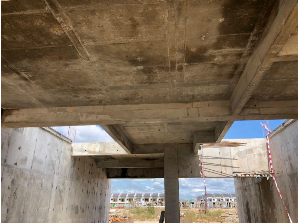
Figure 59: Image shows exposed soffit beams of 1st floor beam after opening of aluminium formwork.
