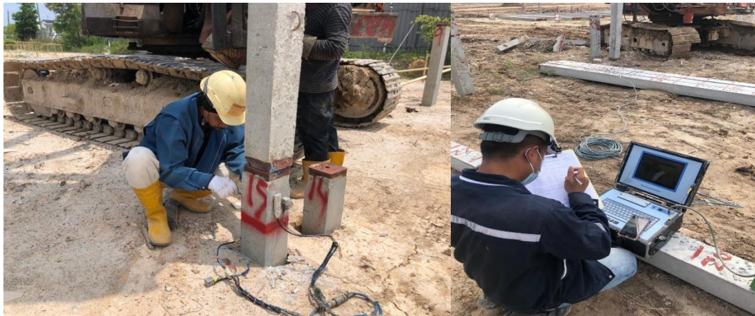
Figure 10: Image (Left) shows 2 sets of accelerometer gauges bolted on pile & image (Right) shows PDA equipment for PDA testing.
