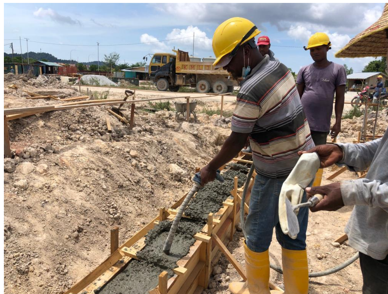
Figure 22: Image shows the vibration of concrete during casting using an immersion vibrator.
