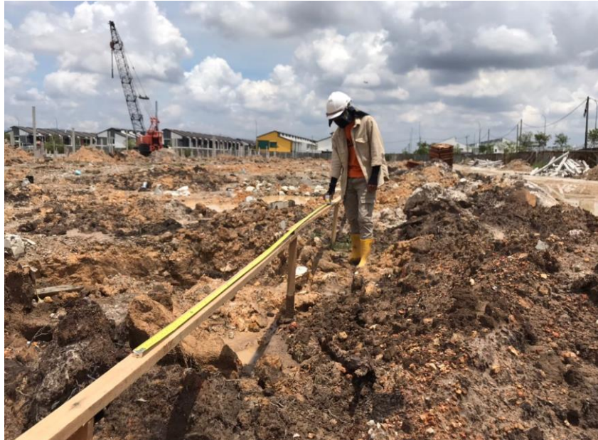
Figure 14: Image shows 'checking' of boundary rails that was marked with the intended pile positions.
