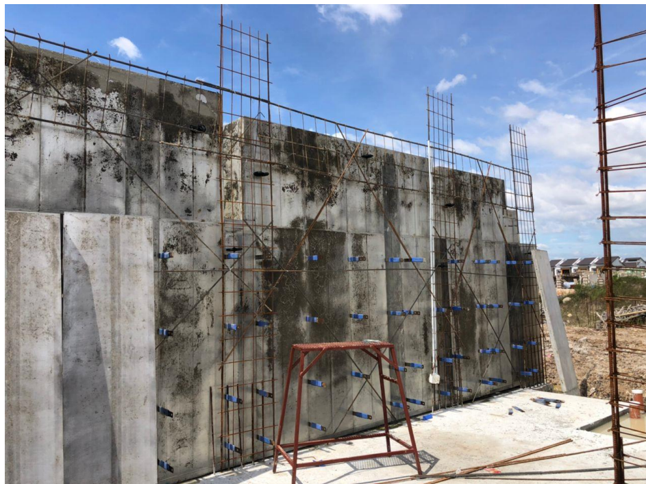
Figure 53: Image shows the complete installation of BRC and reinforcement bars for R.C wall.
