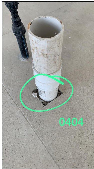
Figure 24 : Incorrect Measurement And Cut The Tiles
