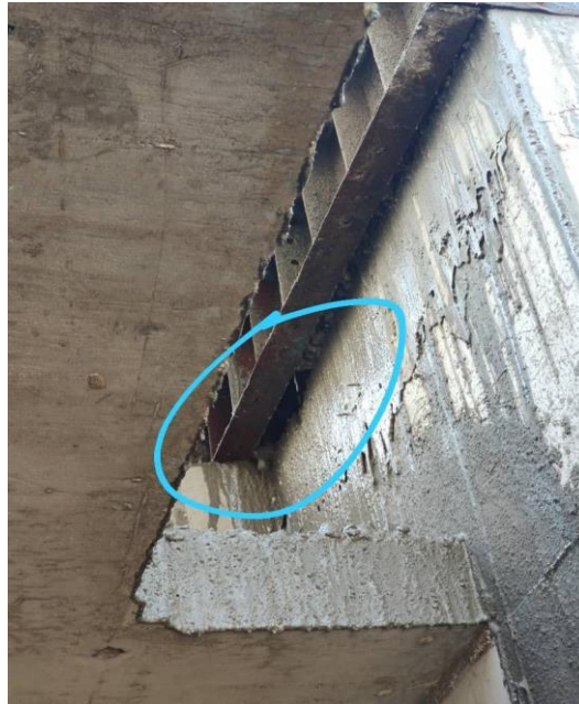
Figure 3.39: Concrete water leakage due to uneven surface level of slab
