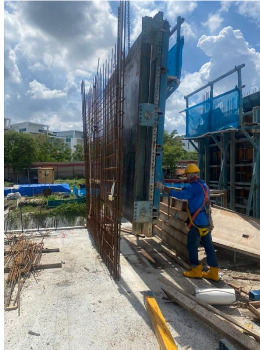
Figure 3.17: Shows the installation of shear wall using the simple form work system on one side
