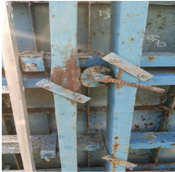
Figure 3.38: Rusted Tie Nuts and Bended Hollow (Bracing)
