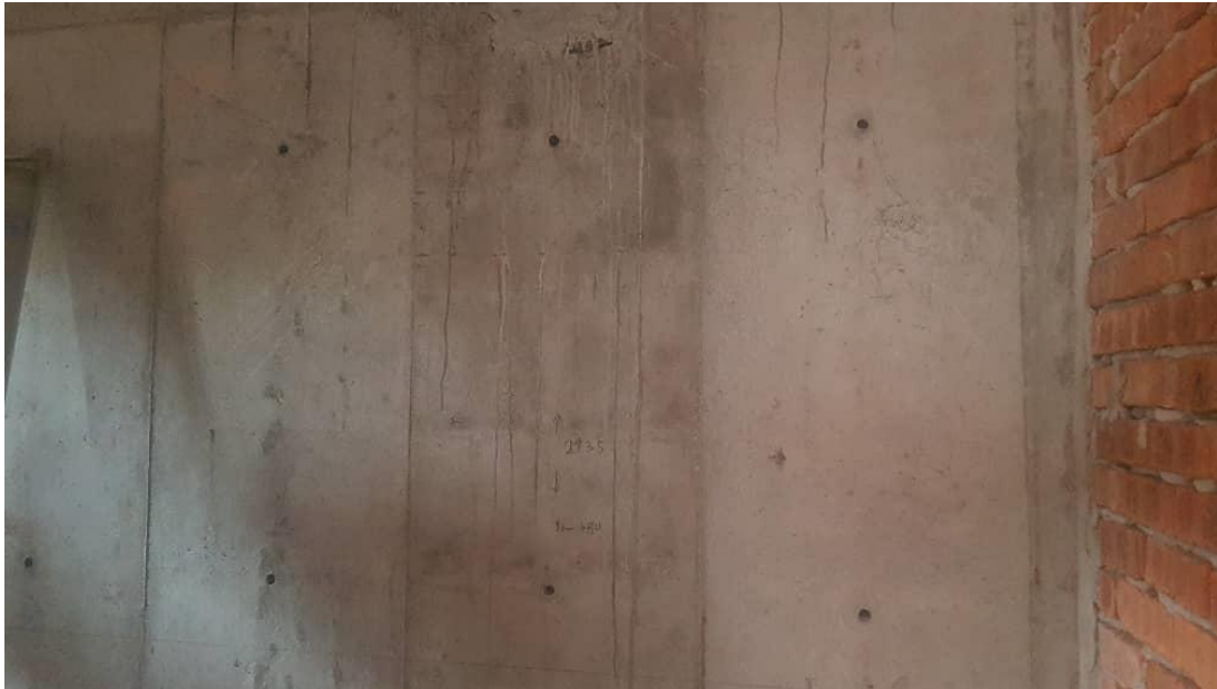
Figure 3.36: Holes left by tie rods on the surface of shear walls
