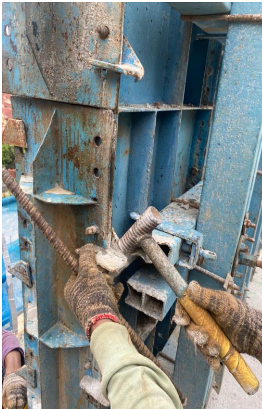
Figure 3.20: Shows the installation of lock pin to tighten the pair of ganged formwork panels
