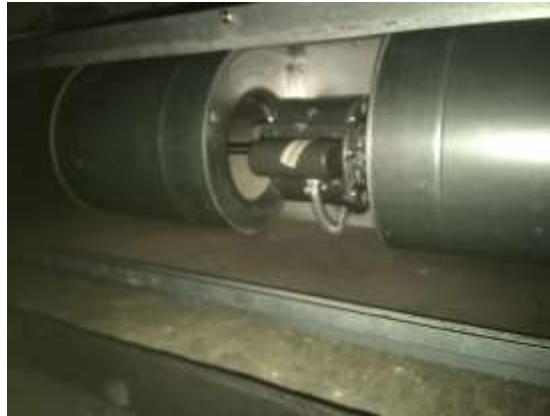
Figure 3.50 : Motor blower air conditioner
