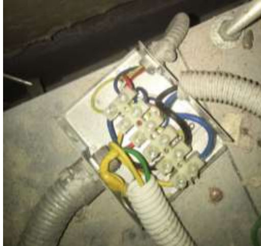
Figure 3.51 : Air conditioner wiring
