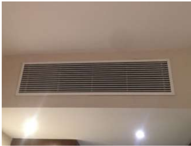
Figure 3.16 : Air conditioner grill
