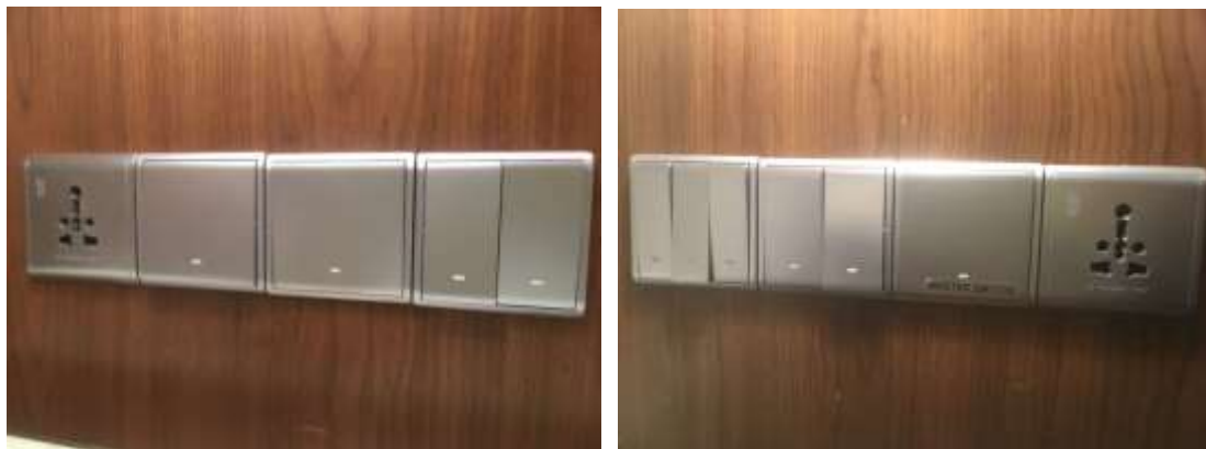
Figure 3.36 : Switch at bedside
