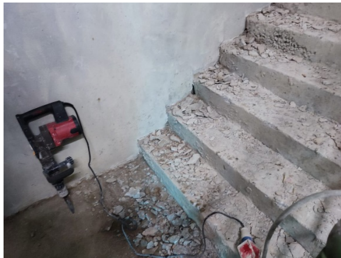
Figure 19: Hacking Work For Honeycomb Defect
