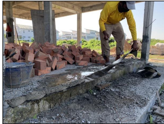
Figure 22: Every bottom layer of brick needs to put Damp Proof Course (DPC)
