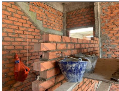
Figure 31: 'Teething' at intersection joint
