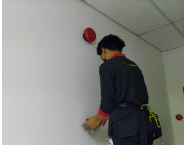
Figure 14: Fire alarm bell
