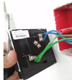
Figure 23: Electric wire connect to manual call point
