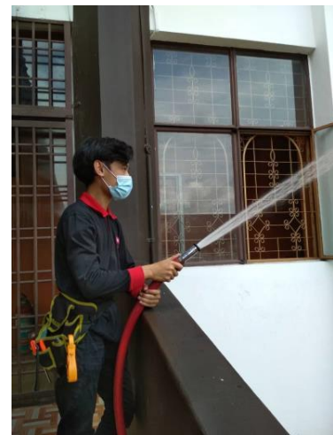
Figure 19: Testing hose reel
