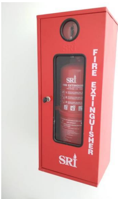
Figure 13: Portable fire extinguisher
