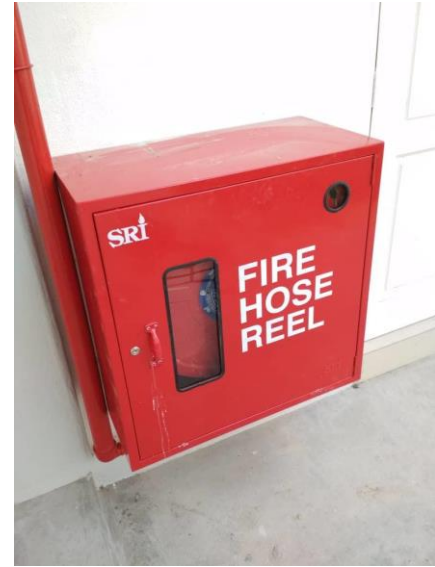
Figure 8: Fire hose reel
