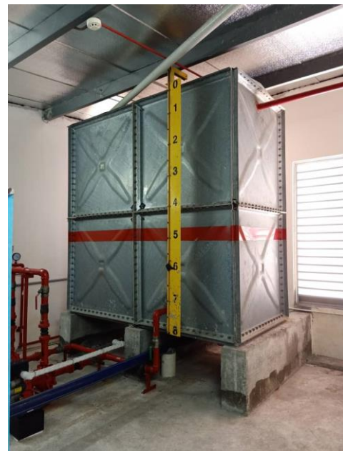
Figure 9: Fire water storage tank upper level 1
