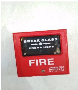
Figure 15: Manual break glass alarm
