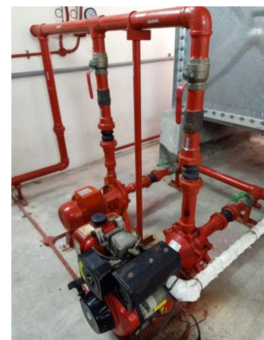
Figure 20: On duty and standby pump ready to use
