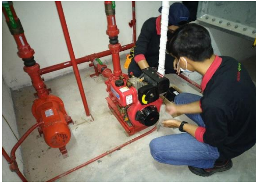
Figure 10: On duty and standby duty pump
