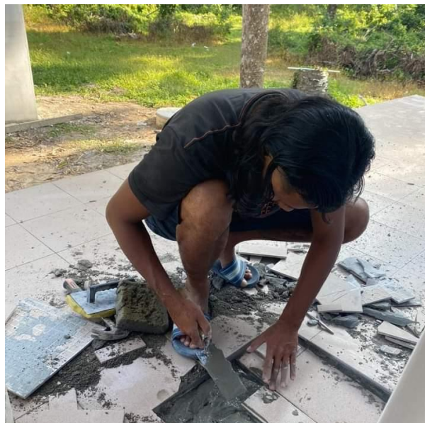
Figure 3.15 one of the worker unplug the wrong tile
