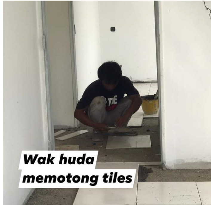
Figure 3.17 Inappropriate method of cutting tile
