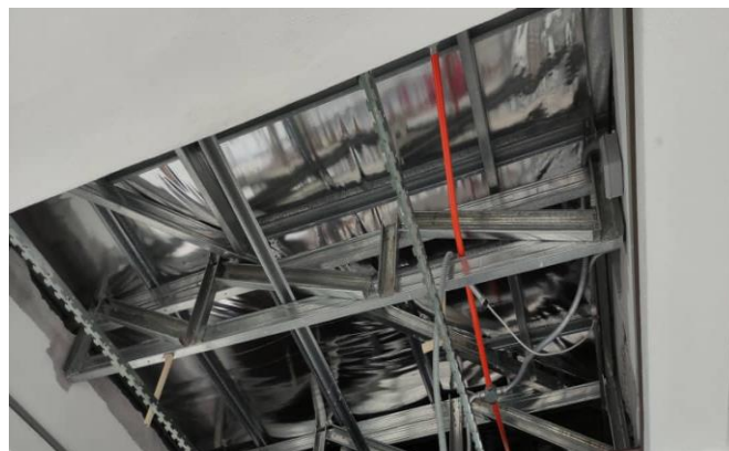
Figure 3.3.6(2) Main keel have been installed and ready to hold the aluminium panel
