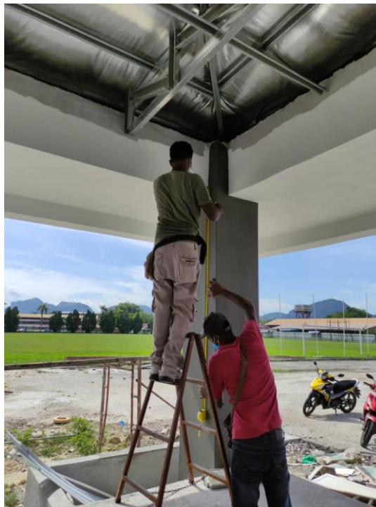
Figure 3.4(3): Last day of working. The worker in the picture measuring height before installing ceiling
