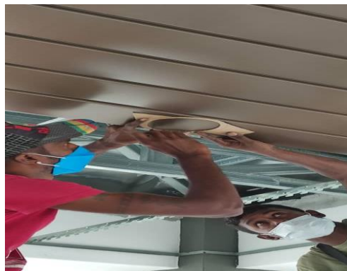
Figure 3.3.7(2) Worker is making a round hole for light features and cut it for installation of light features later
