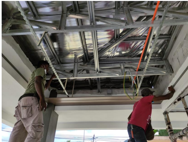
Figure 3.4(1) Day 1 of working. Worker installing aluminium strip ceiling on the front of the guard house
