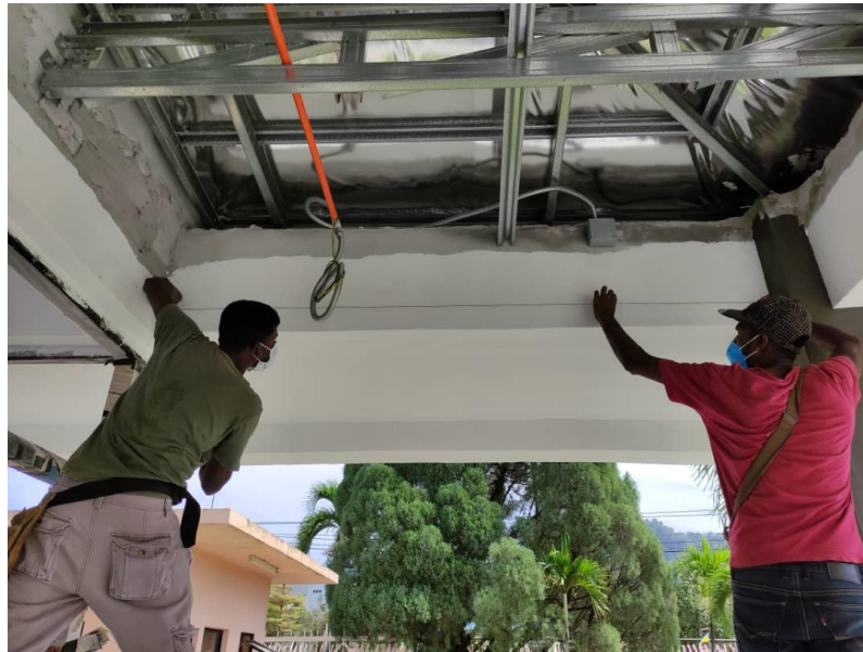
Figure 3.4(2) Day 2 of working. Worker continue installing ceiling and the picture above is the worker is marking using a string
