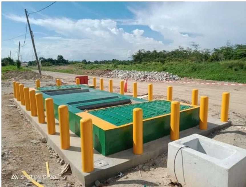
Figure 3.34: Compact substation finished
