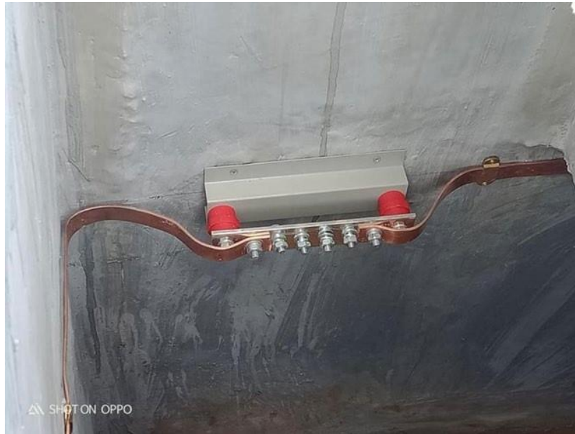
Figure 3.25: Complete installation earthing system in compact substation
