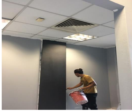
Figure 3.2.17: The second coating paint for the column Source: Fadlhlin Engineering project document
