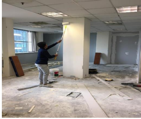
Figure 3.2.15: The first coating paint for the column Source: Fadhlhin Engineering project document
