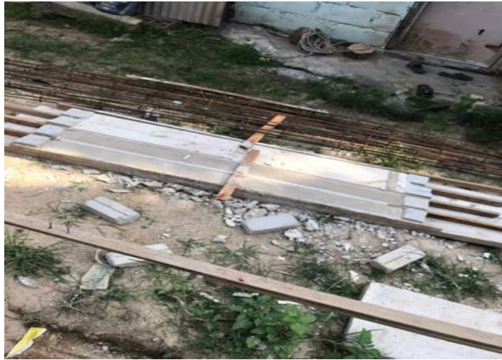
Figure 3.10: The lintels that used as a load support at the top of opening parts.
