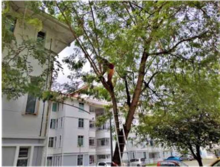
Photo 2.12 Pruning trees that approaching the building structure, shading, and other obstruct access needed
