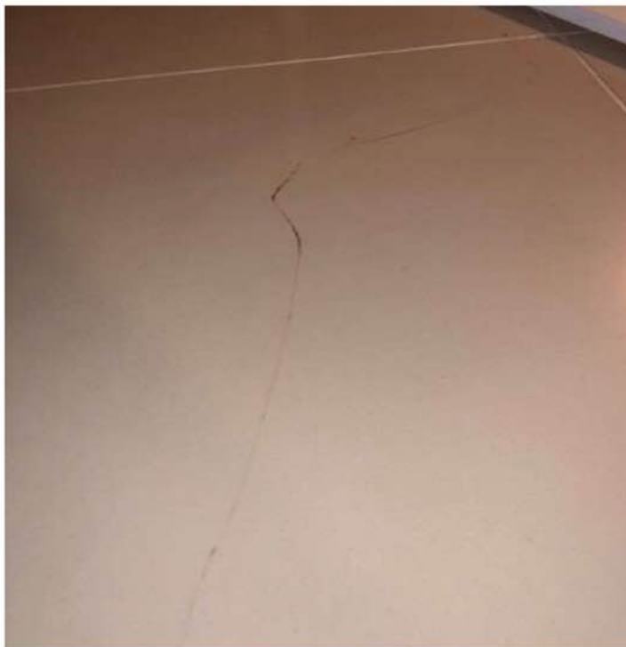
Photo 3.38 Scratches on Porcelain Granite Tile
