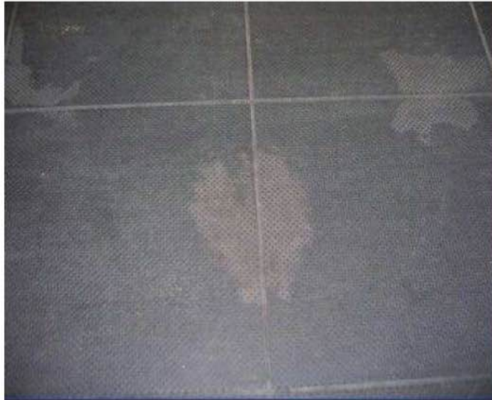
Photo 3.39 Stain on Porcelain Tiles
