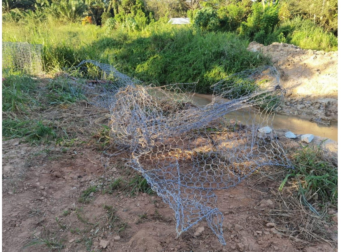
Figure 3.5 the broken cage effect from landslide.
