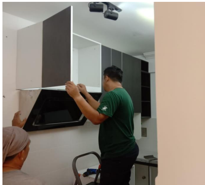
Photo3.11: The installation of custom-made kitchen cabinet which the services provided by Dekad Wangsa Sdn Bhd at PPA1M, Putrajaya
