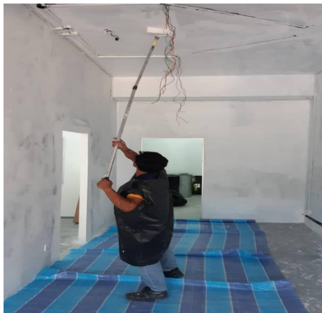
Photo 3.9: The uses of canvas while painting the ceiling to protect the floor
