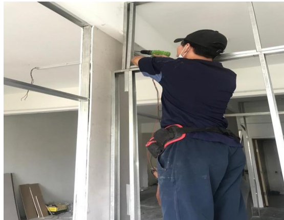
Photo 3.12: The installation of partition board for making the separate room for office at Batu Caves
