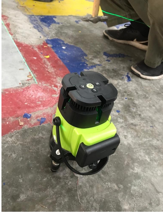
Photo 3.14: Professional automatic laser line used to make sure the partition wall is straight horizontally and vertically
