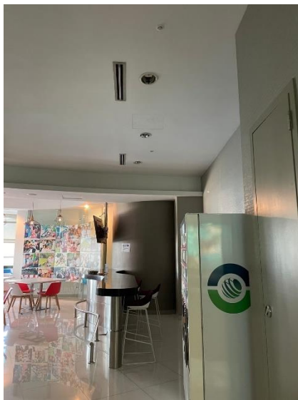
Figure 3.21 Broken Lamp at Café Area
