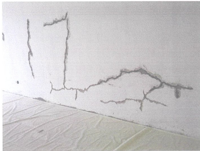
Photo 3.3.1.1 cracking at the wall
