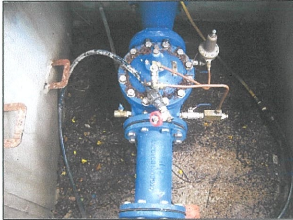
Gambarfoto 4.9 : “Pressure Reducing Valve” (PRV)
