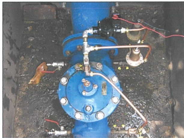
Gambarfoto 4.10 : “Pressure Reducing Valve” (PRV)
