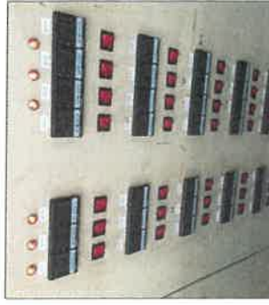
STEP 4: TURN OFF ALL HEATER GH & MH
