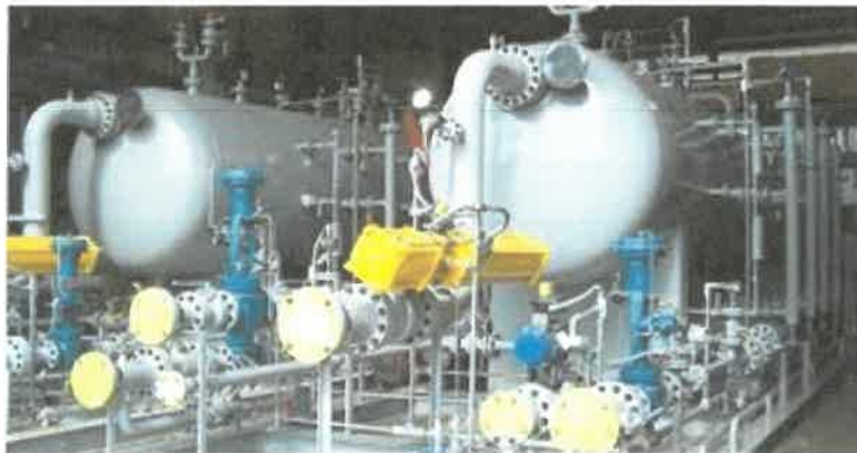
Figure 4.9: Physical photo of oil-water static separation tank
