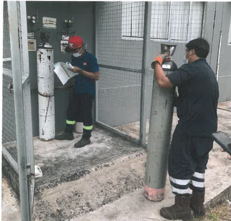
Figure 13 Changing new nitrogen gas
