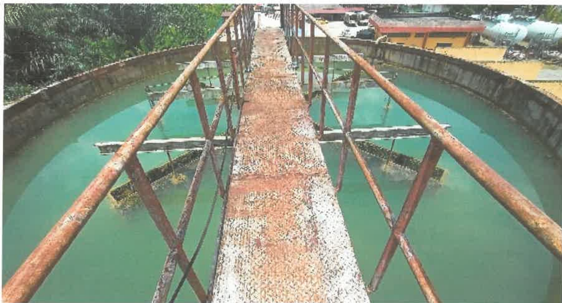
Figure 3.5.2 Sedimentation Tank in Kuala Pilah Water Treatment Plant
