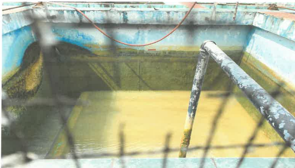
Figure 3.7.2 Rapid Sand Filter in Lakai Water Treatment Plant
