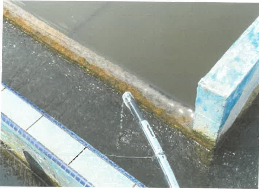
Figure 3.6.1 Intermediate dosing in Kuala Klawang Water Treatment Plant
