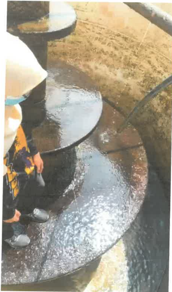
Figure 3.3.1 Aerator and pre-dosing of Pedas Baru Water Treatment Plant
