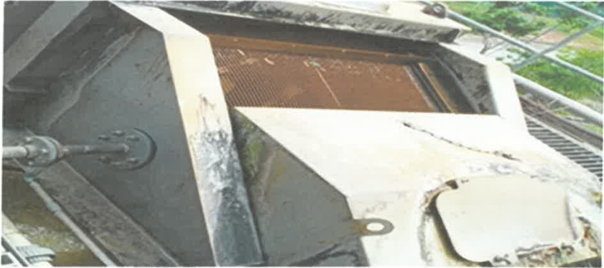
Figure 3.1.3 Rotary Drum Screening in Sawah Raja Water Treatment Plant
