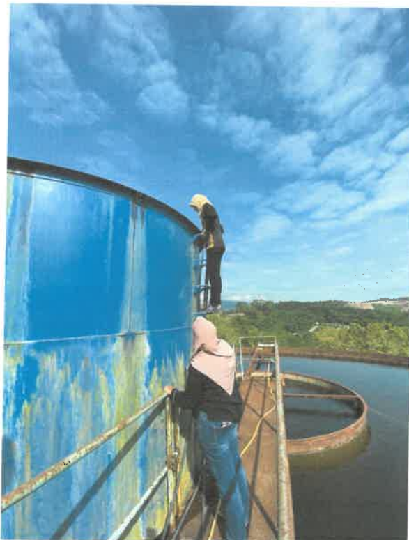
Figure 4.5.3 Checking aerator before calibration
