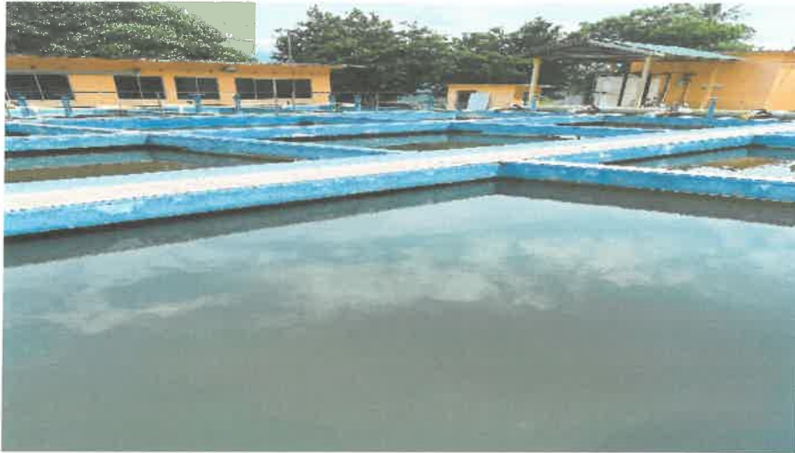
Figure 3.5.1 Sedimentation Tank in Kuala Klawang Water Treatment Plant
