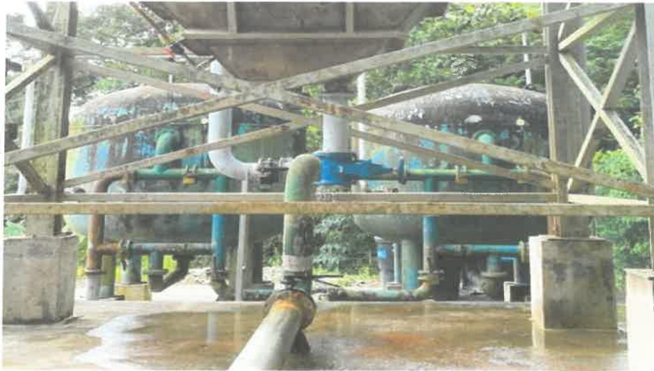
Figure 3.7.1 Pressure Filter in Ulu Bendul Water Treatment Plant
