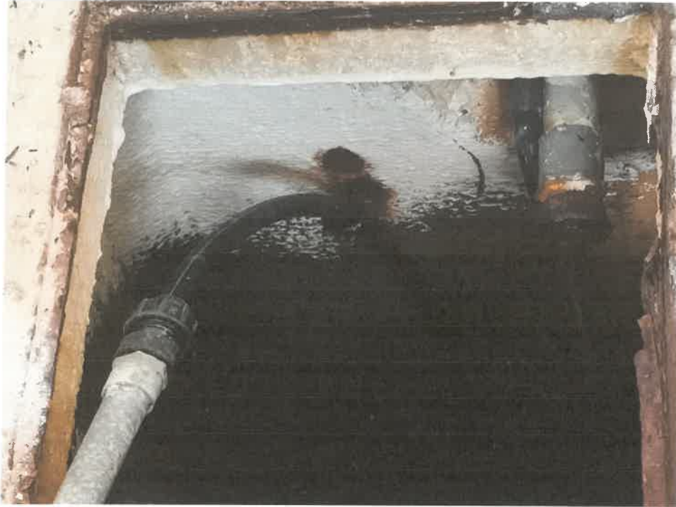
Figure 3.8.1 Fluoride Dosing in Kuala Klawang Water Treatment Plant
