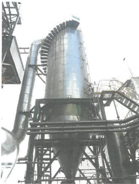
Figure 6.9: Semi Dry Reactor
