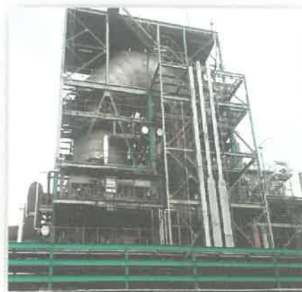
Figure 6.2: Secondary Combustion Chamber
