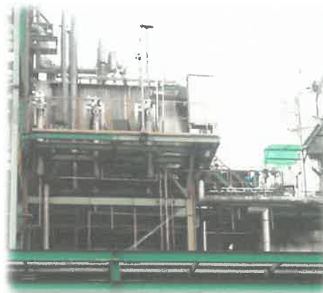
Figure 6.3: Boiler & Air Pre-Heater
