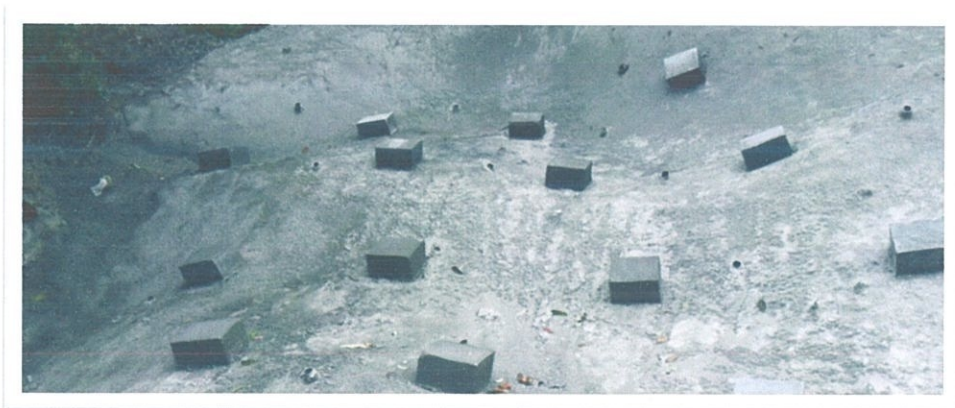
Figure 3.3.7.1: Nail pad has been construct proper tabulation as per recommended based on its design by the structural engineer
