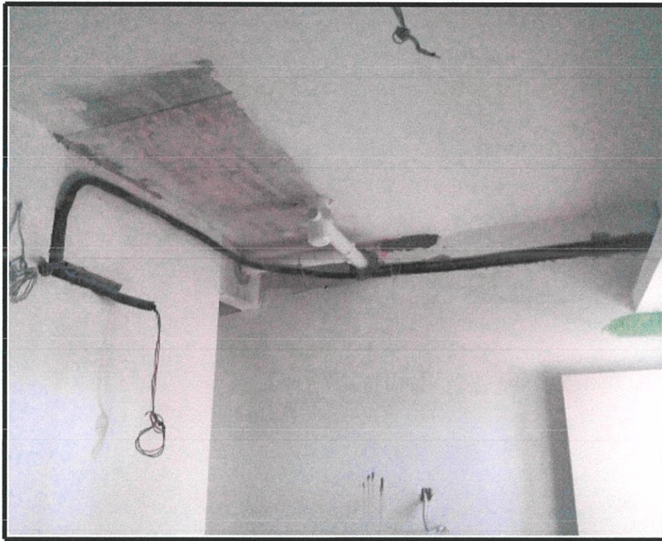
Photo 3.9 included pipe in the wall
