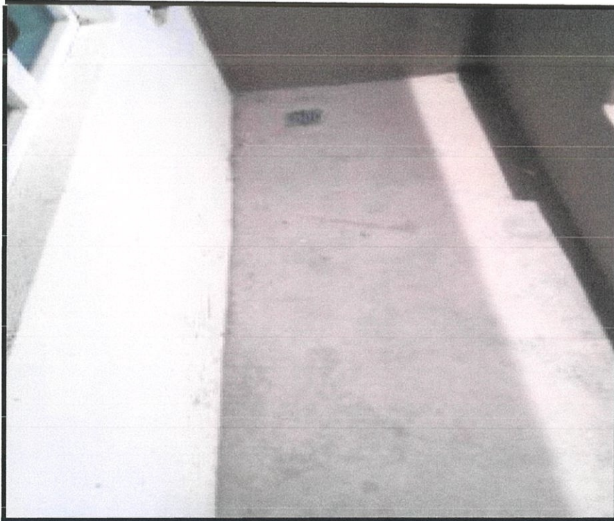
Photo 3.12 place of condenser
