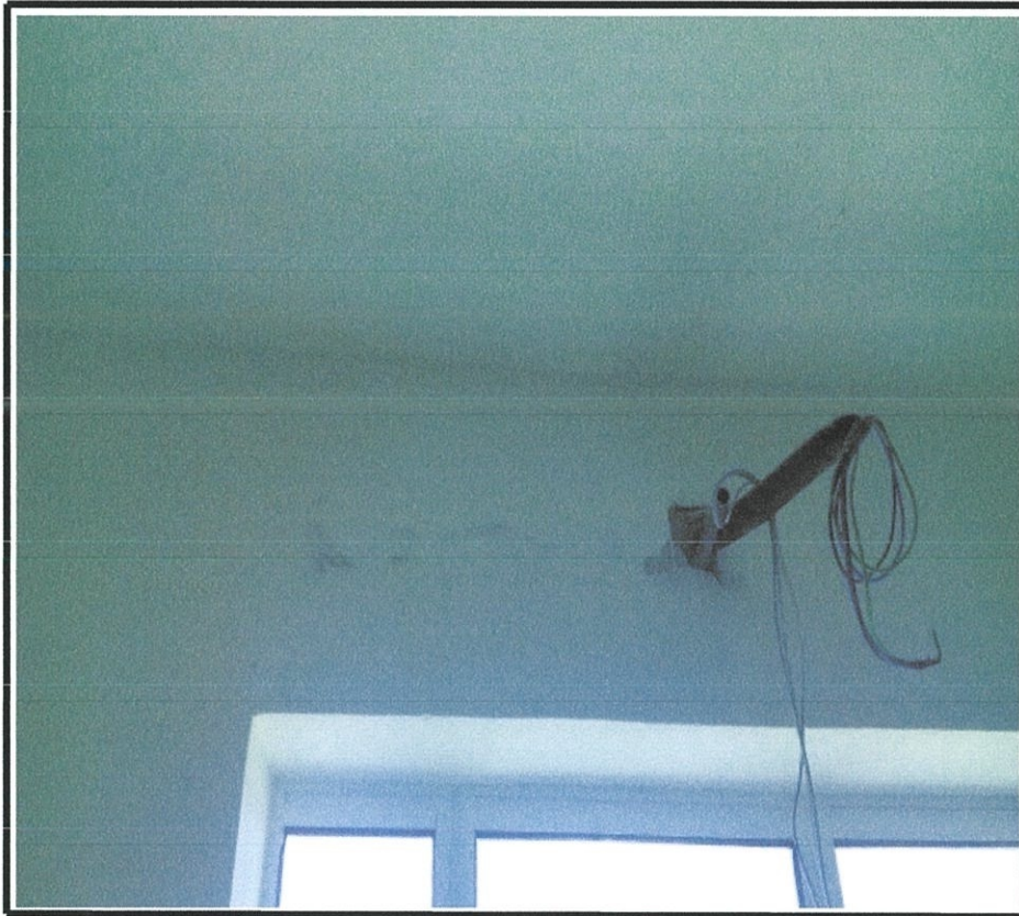
Photo 3.8 hole at wall
