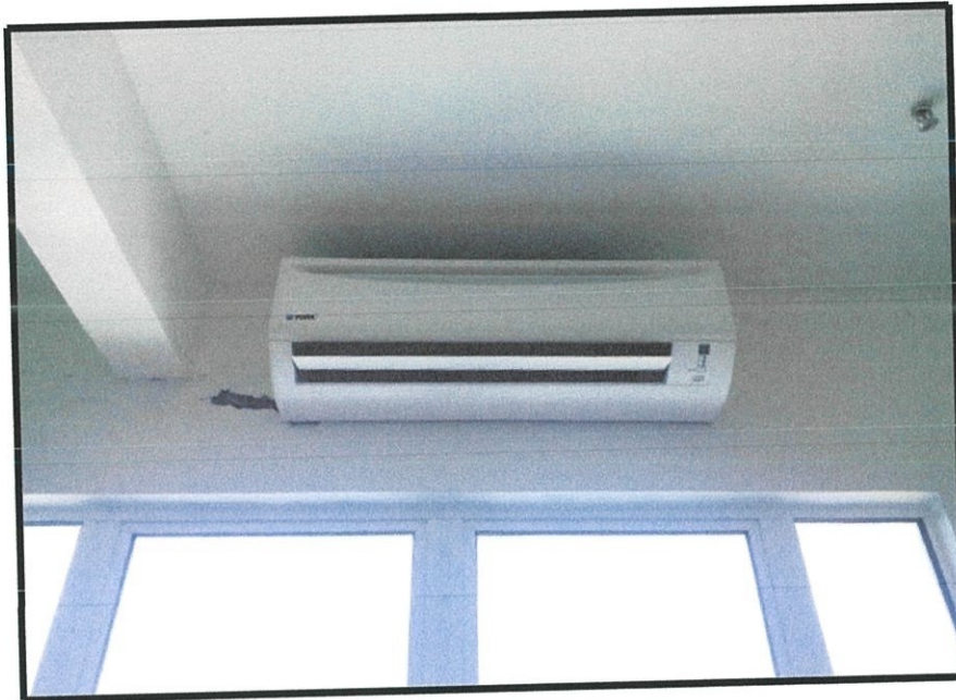
Photo 3.6 split unit indoor
