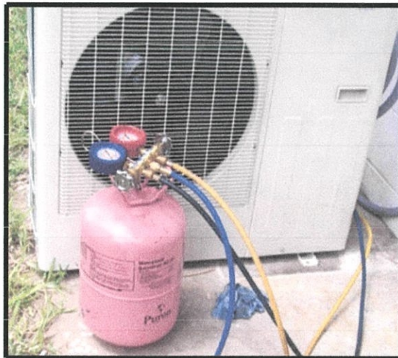
Picture 3.31 gas refrigeration
