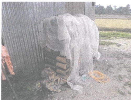
Photo3.18 Cement not over cover.
