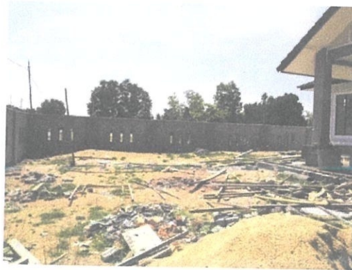
Photo 3.13 Messy layout at site build.
