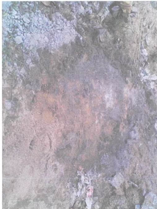
Photo 3.4 Cement mixing place on soil can cause wastage to quantity of mortar.
