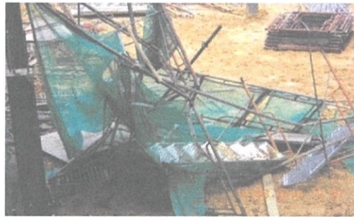
Photo 3.14 Staging not tough enough.
