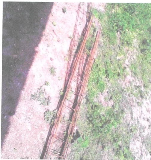
Photo3.12 Reinforcement for roof beam not be placed at right place.
