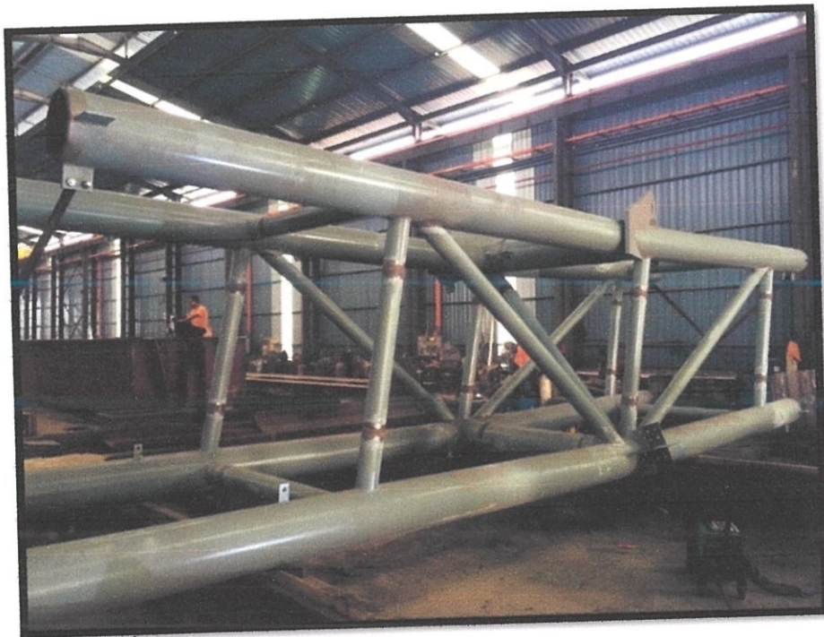
Photo 3.1 One segment which is complete being combined and waiting for welding works.
