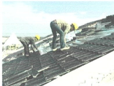
Photo 3.26: Roof installations without any safety.
