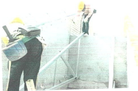
Photo 2.27 : No ladders use.
