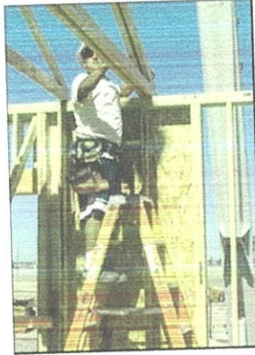
Figure 3.5: Platform ladders can be set up inside a structure and used to install roof trusses.
