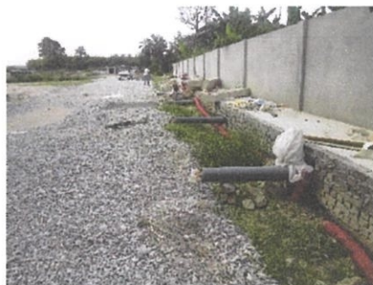
Photo 3.14: Polyvinyl chloride (PVC) pipe type for drain is installed first before kerb
