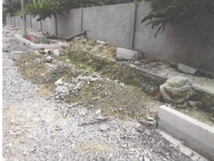
Photo 3.16: Kerbs undergo damages because of digging work.
