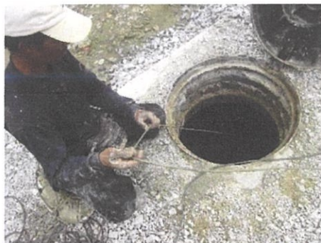
Photo 3.17: crusher run had penetrate drain and cause blockage
