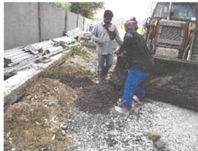
Photo 3.15: Worker had make an error by changing the actual place of kerb that need to be install
