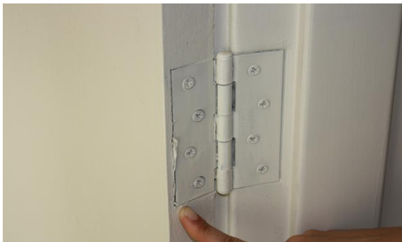
Figure 7: Example of defect
