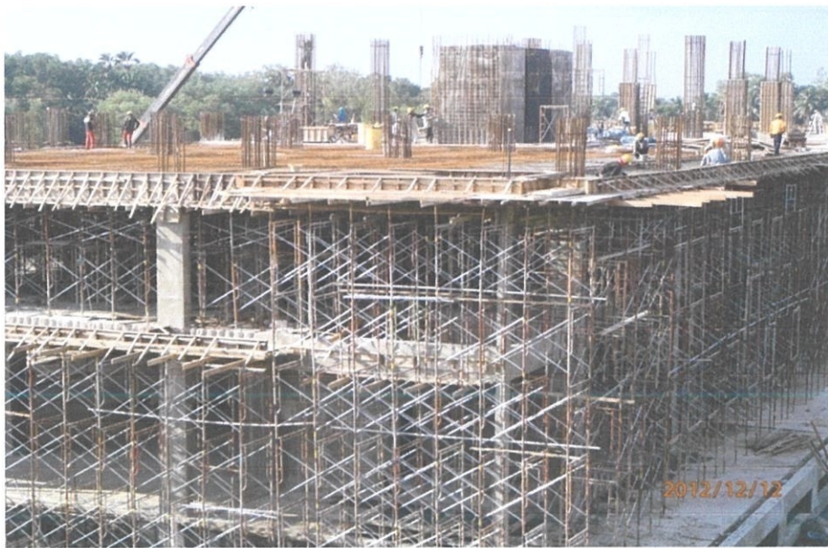
Picture 2 : Scaffolding Frames
