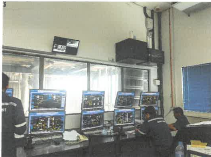
CONTROL ROOM OF OLEO DEPARTMENT
