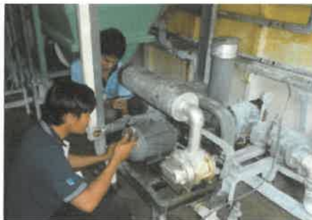
Figure 5 maintenance crew to service
