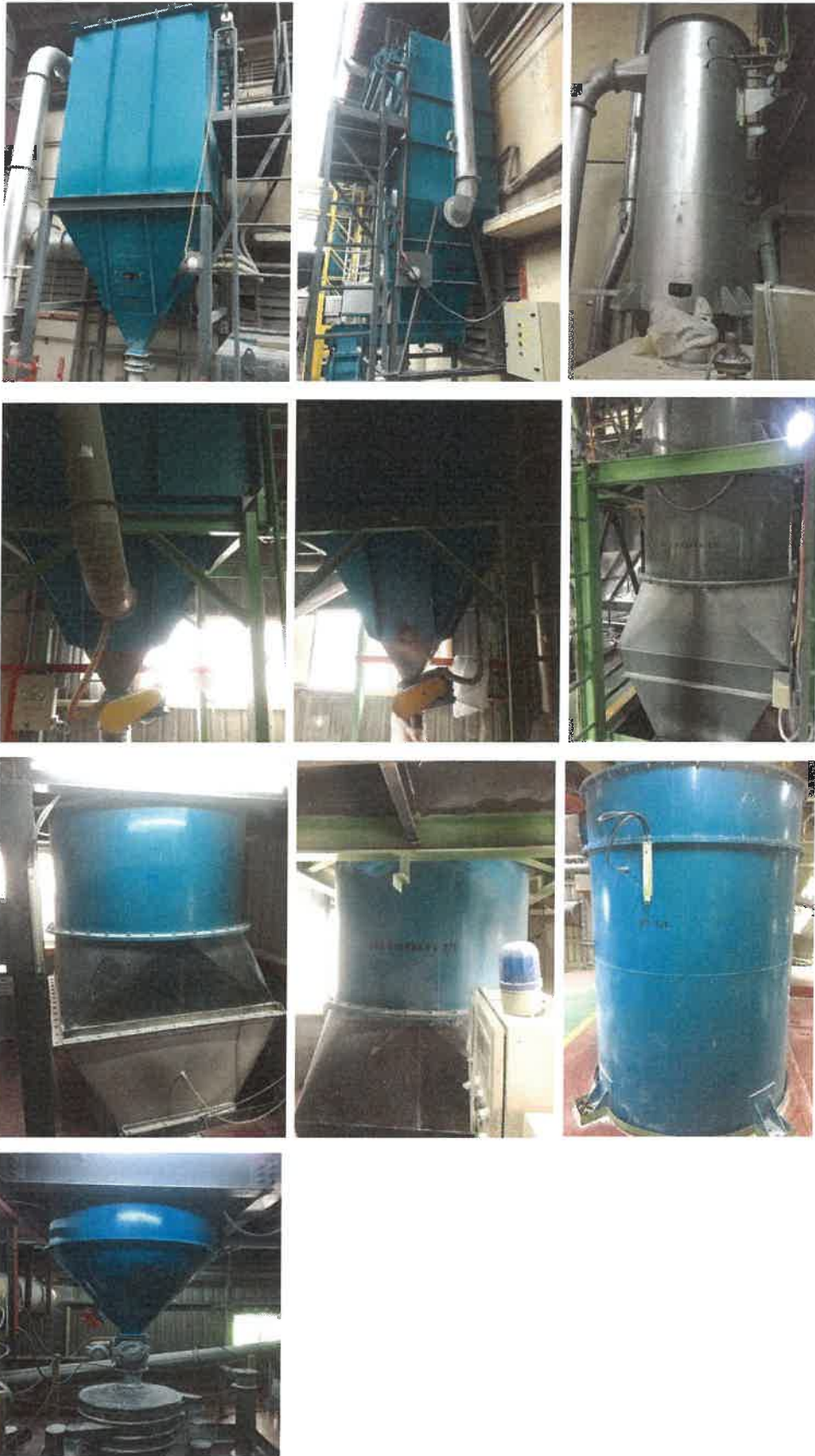
Figures 21: Pictures about the equipment (From top left to right- DC 2 SL, DC 3 SL, DC 4 SL), ( From middle left to right- DC 1&2 DF, DC 3 DF, HS 1 DF), ( From middle left to right- HS 2 DF, HS 3 DF, DF 5 DC), ( Bottom- Transfer silo DF 5)
