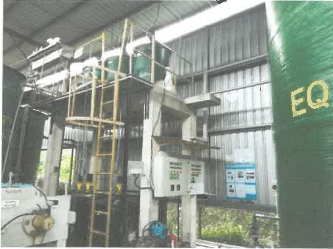
Figure 2: The Wastewater Treatment Plant at Vegeta Manufacturing Sdn Bhd.
