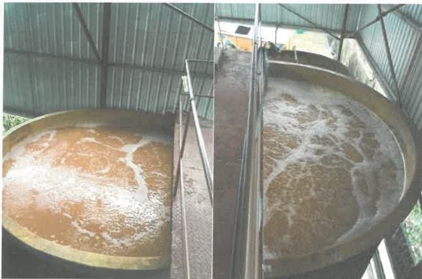
Figure 3: The aeration tanks (Left side: aeration tank 2, Right side: aeration tank 1)
