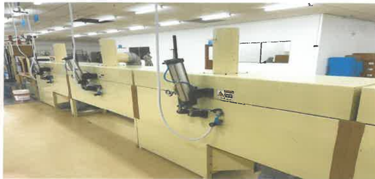
Figure 15: Chamber for Heating Process
