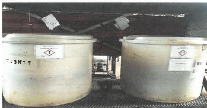
Boiler Water Chemical Tank
