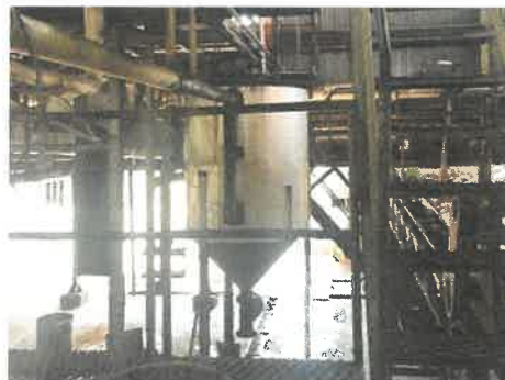
Sand Trap Tank
