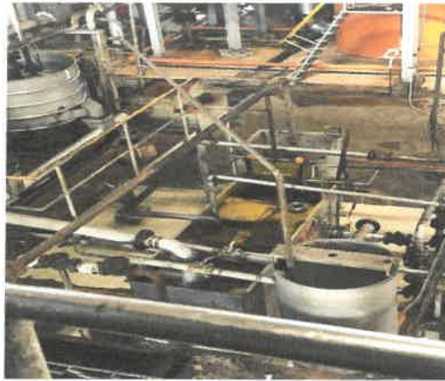
Diluted Crude Oil Tank
