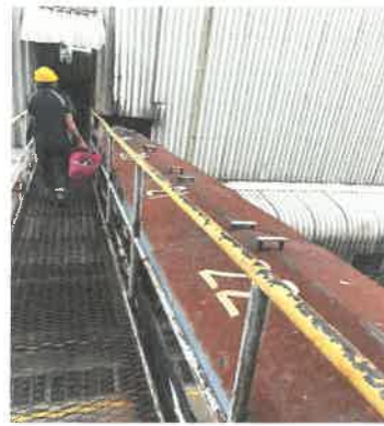
Cake Breaker Conveyor
