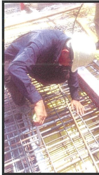
Photo 3.30 The supervisor measure the height of tendon from the surface of formwork
