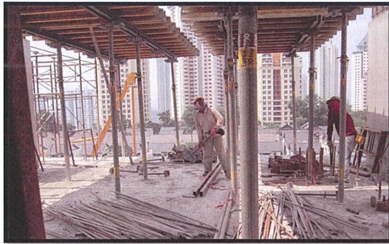
Photo 3.19 The workers adjust the verticality of the formwork by using a plastic mallet
