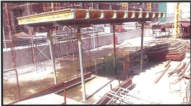
Photo 3.16 The table formwork which prefabricated on the site and ready to set to its using location
