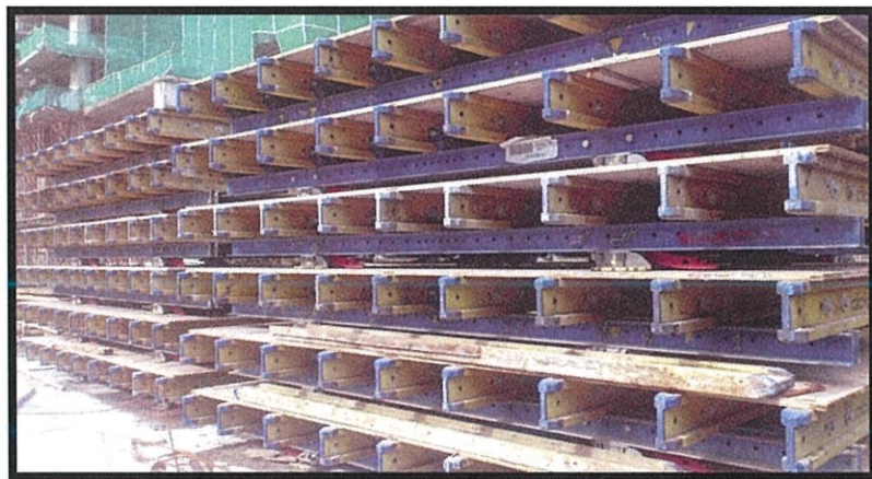
Photo 3.14 Table platforms of Doka Formwork which still on stack before mounted process
