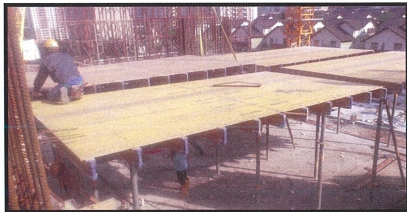
Photo 3.18 The workers fix the table formwork and arrange it to be in straight position
