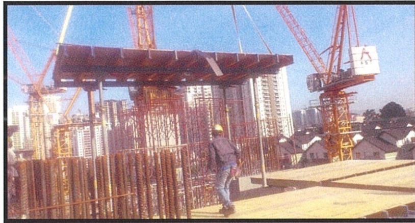
Photo 3.17 The tower crane used as a transport to carry the table formworks to its using location
