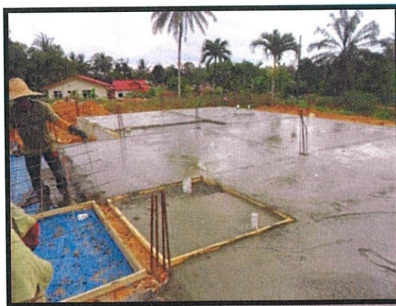
Figure 15: Concrete on the Floor Slab
