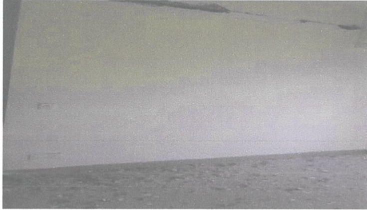
Picture 3.2: Wall Crack
