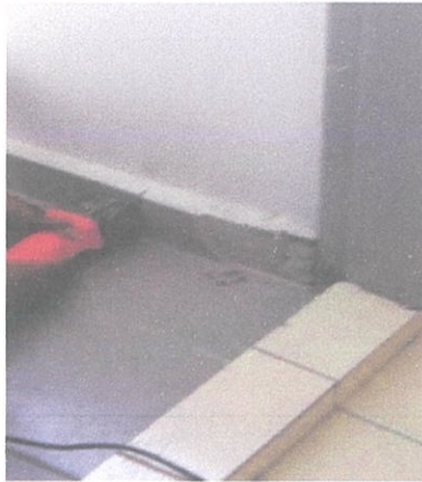
Picture 3.19: Skirting Tiles Broken
