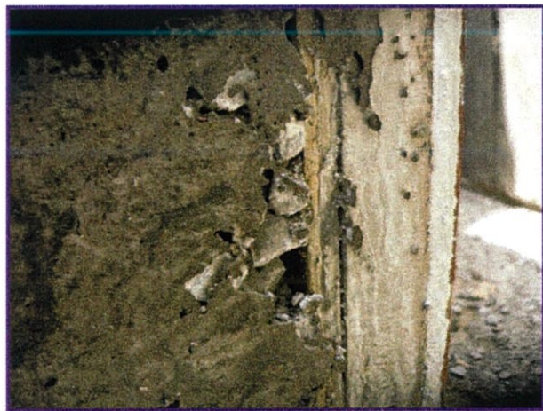
Photo 4.34: Honey combing on the surface of wall.
