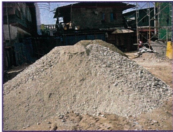
Photo 4.14: The crusher run is put in a temporary place on site before use
