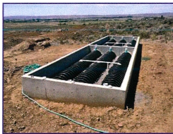
Figure 3.9: Reticulation aerobic sand filters
