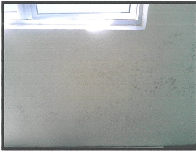
Photo 3.3.4 Mildew of Paint Surface
