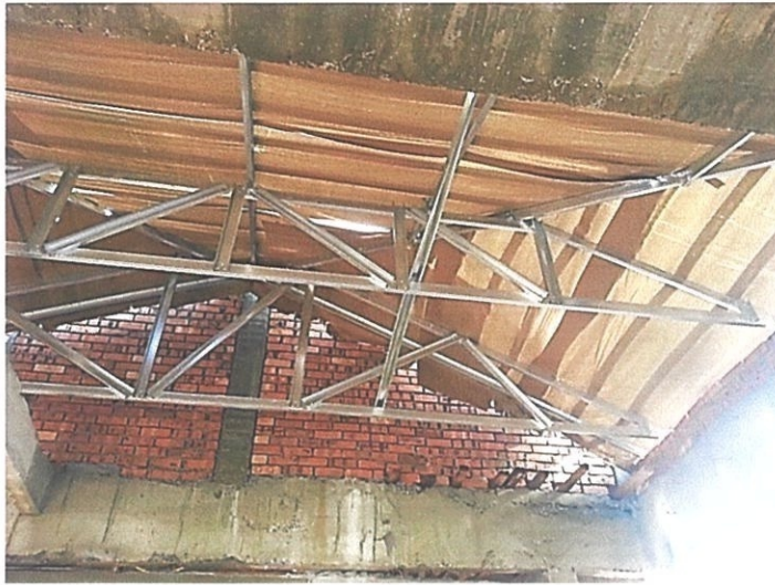
Photo 3.3.2.12 Combination of Step down Hip and Hip Truss in Roof Construction of Bungalow House in Taman Dato' Wan, Ampangan
