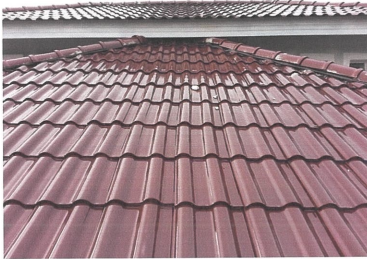
Photo 3.3.4.12 After the Installation of Roof Tiles for Pitched Roof in Roof Construction of Bungalow House in Taman Dato' Wan, Ampangan
