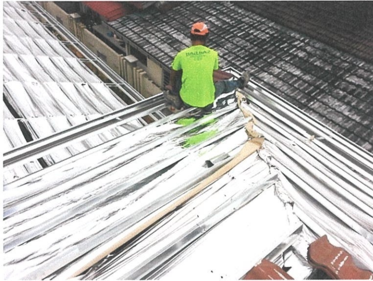
Photo 3.3.4.10 Before the Installation of Roof Tiles for Pitched Roof in Roof Construction of Bungalow House in Taman Dato' Wan, Ampangan
