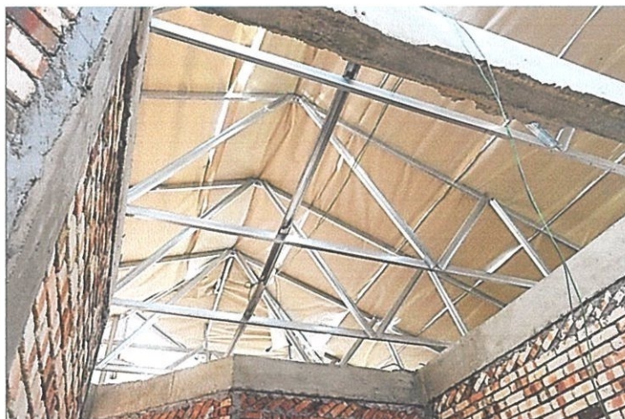
Photo 3.3.2.8 Belgian Truss of Bungalow House in Roof Construction of Bungalow House in Taman Dato' Wan, Ampangan
