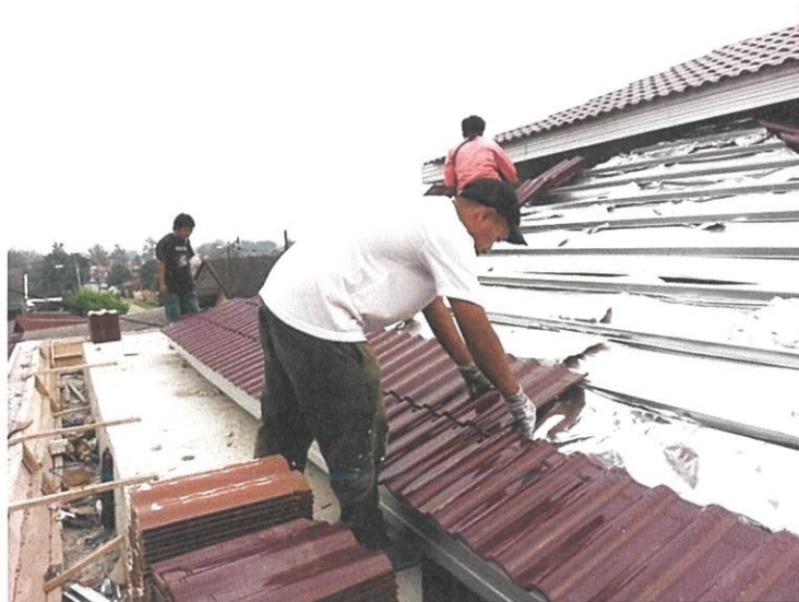
Photo 3.3.4.11 During the Installation of Roof Tiles for Pitched Roof in Roof Construction of Bungalow House in Taman Dato' Wan, Ampangan
