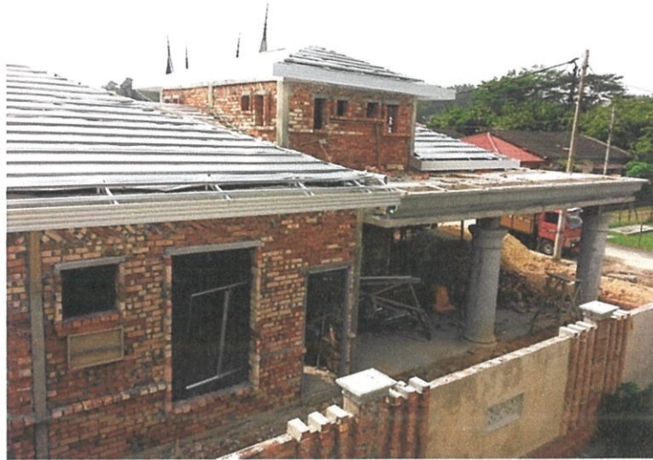
Photo 3.3.4.9 The View of Pitched Roof after the Installation of Roof Batten in Roof Construction of Bungalow House in Taman Dato' Wan, Ampangan
