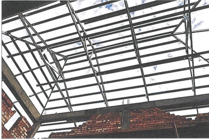
Photo 3.3.2.4 Queen Post Truss in Roof Construction of Bungalow House in Taman Dato' Wan, Ampangan
