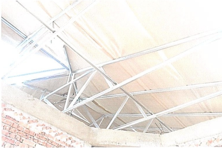
Photo 3.3.4.8 Application of Heat Insulation for Pitched Roof in Roof Construction of Bungalow House in Taman Dato' Wan, Ampangan
