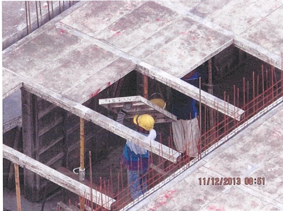
Figure 3.20: Slab Panel are lifting up
