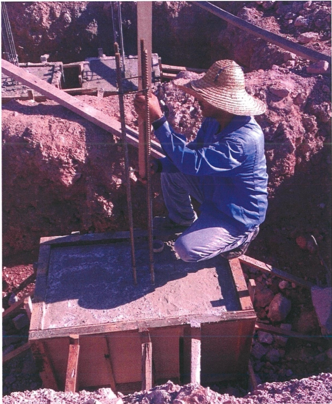
Photo 3.12 A worker marked the level of the column stump and ground beam.
