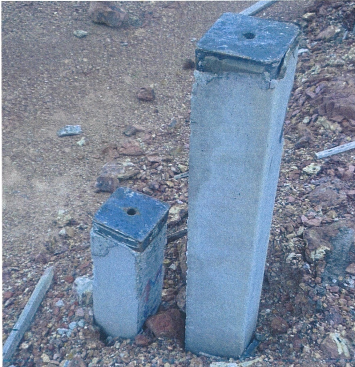
Photo 3.19 Piles on the left was out of alignment. Piles on the right were added to stay in the correct alignment.
