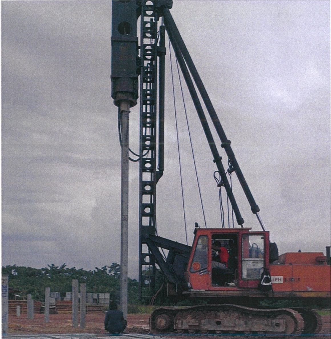
Photo 3.1 The pile machine used at the site, The IPH Hydraulic Piling Hammer.
