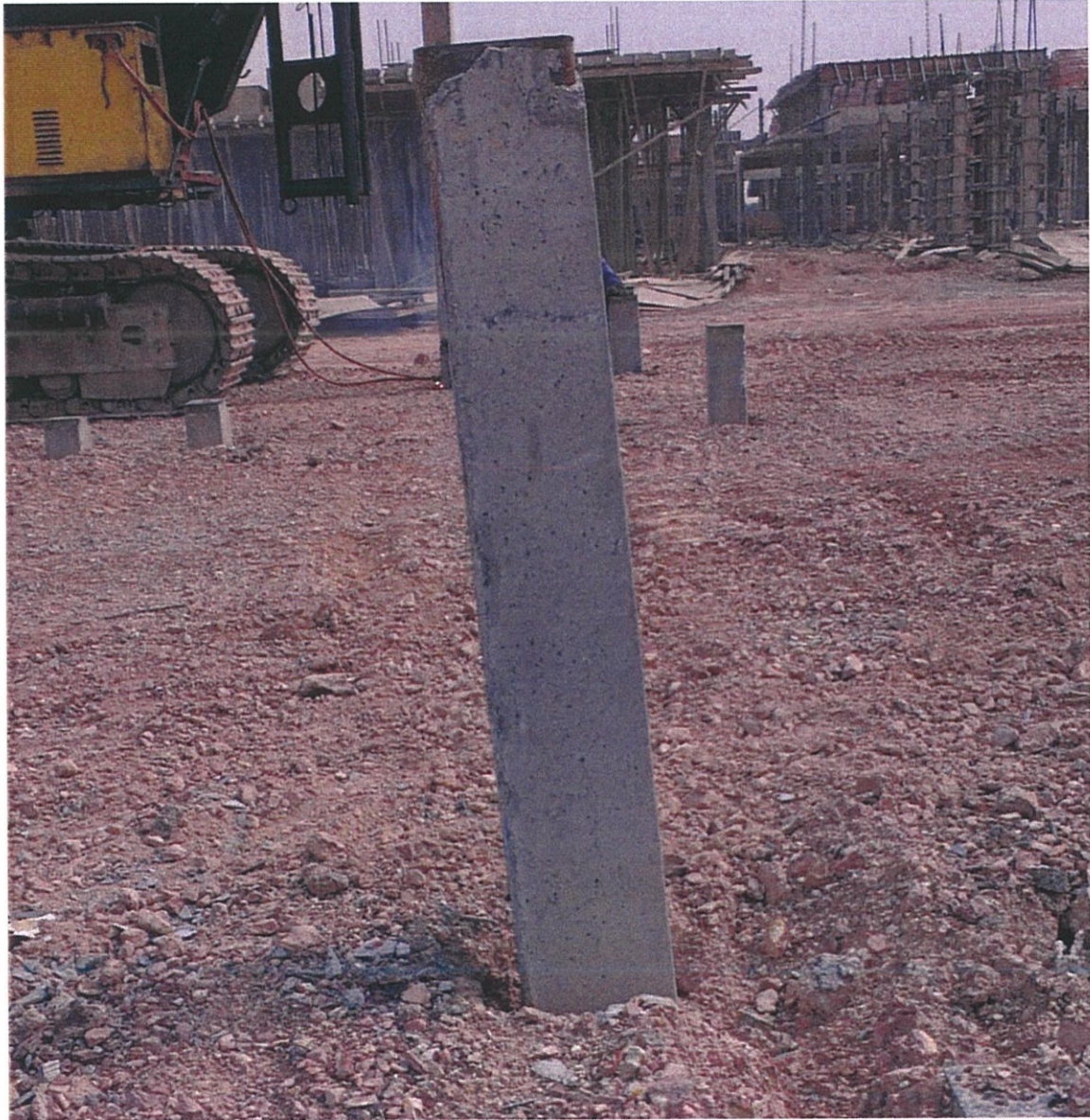
Photo 3.20 The bending of the pile.
