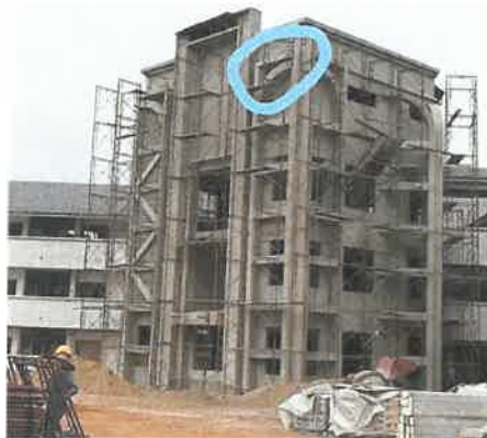
Figure 3.0 shows architect design error made by the sub-contractor
