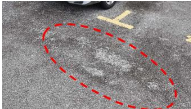
Figure 3.21 Example of uneven surfaces on the road.
