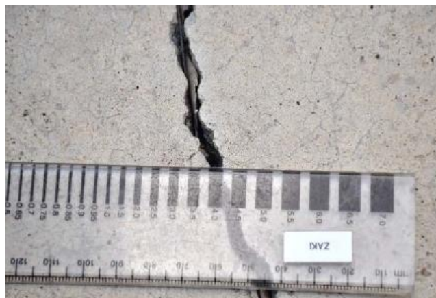
Figure 3.16 Width crack line on the apron using crack gauge
