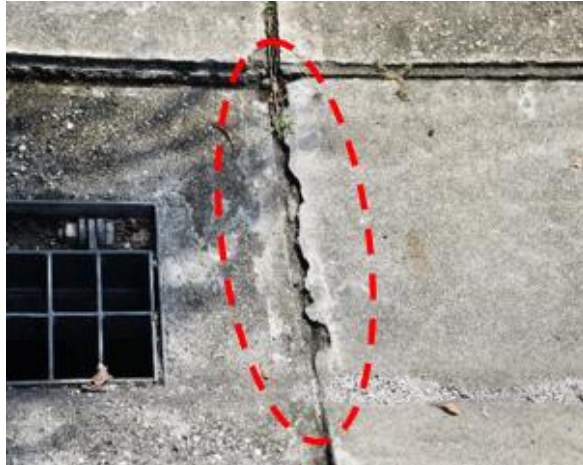
Figure 3.22 Chipped off cement screed on the road drain
