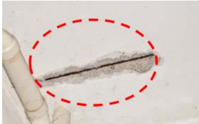
Figure 3.25 Spalled concrete on the soffit slab
