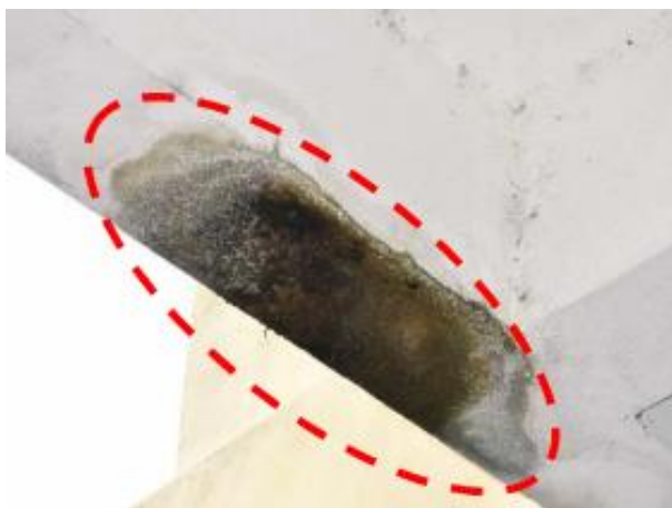
Figure 3.24 Water stain marks on the beam
