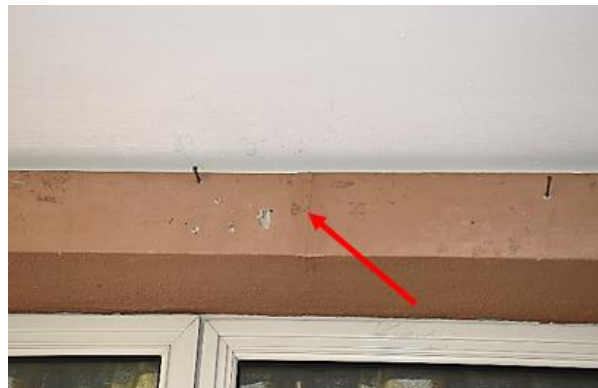
Figure 3.15 Fine crack line on the coping
