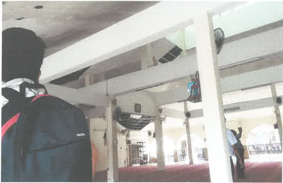
Figure 2.2.3 : Visit places that need to be repaired in the Pusat Islam, Politeknik Sultan Mu,adzam Shah
