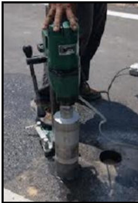
Figure 3.5 : Have a hole in the surface of premix
